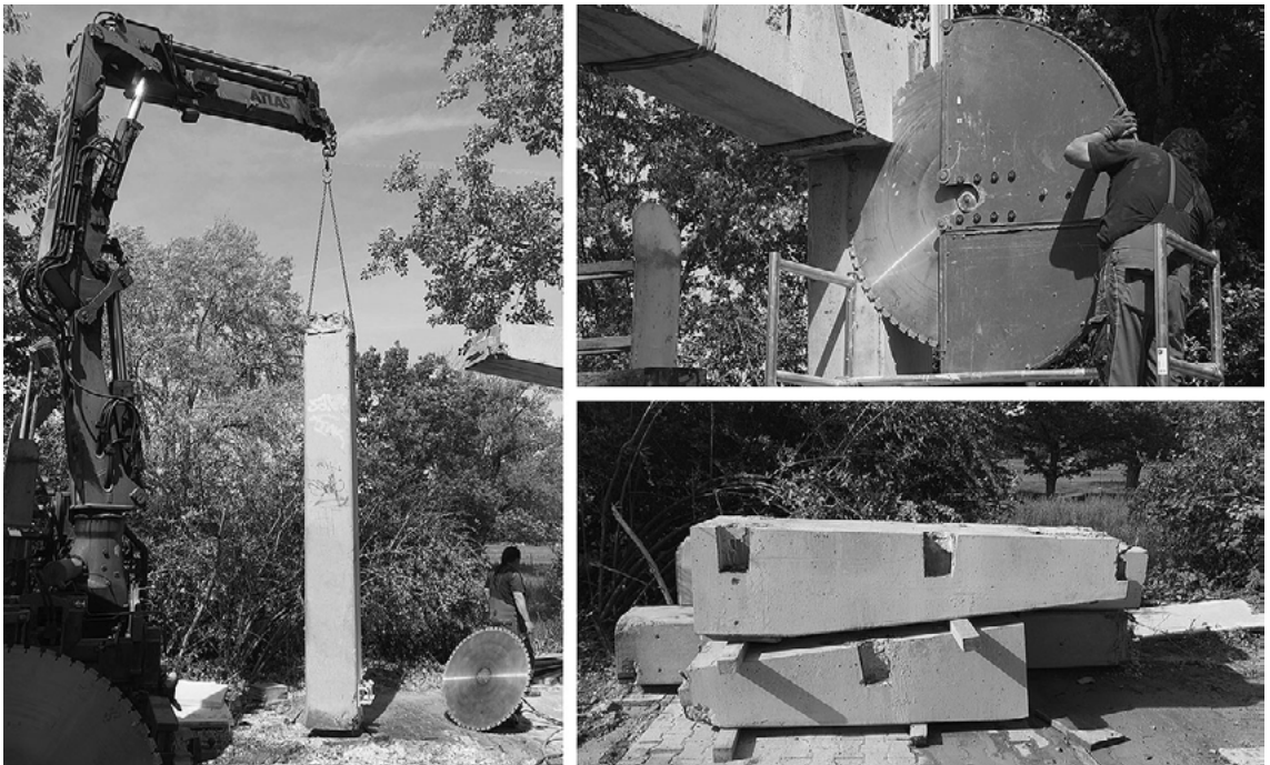
Figure 3. Selective disassembly using a diamond-fitted concrete saw as a proof of the concept of harvesting concrete components for reconditioning and reuse.
