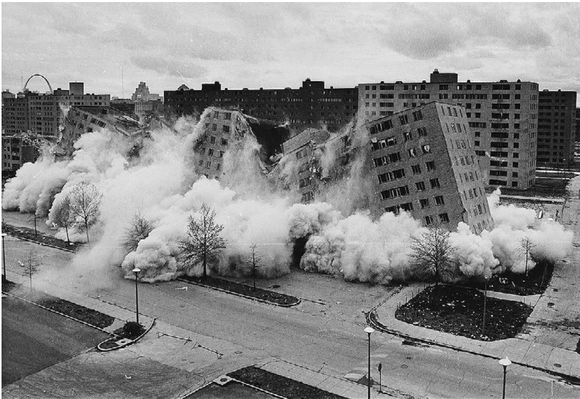
Figure 1. Demolition of Pruitt-Igoe building through controlled blasting on April 21, 1972. (Image credit: U.S. Department of Housing and Urban Development, image placed in Public Domain)
